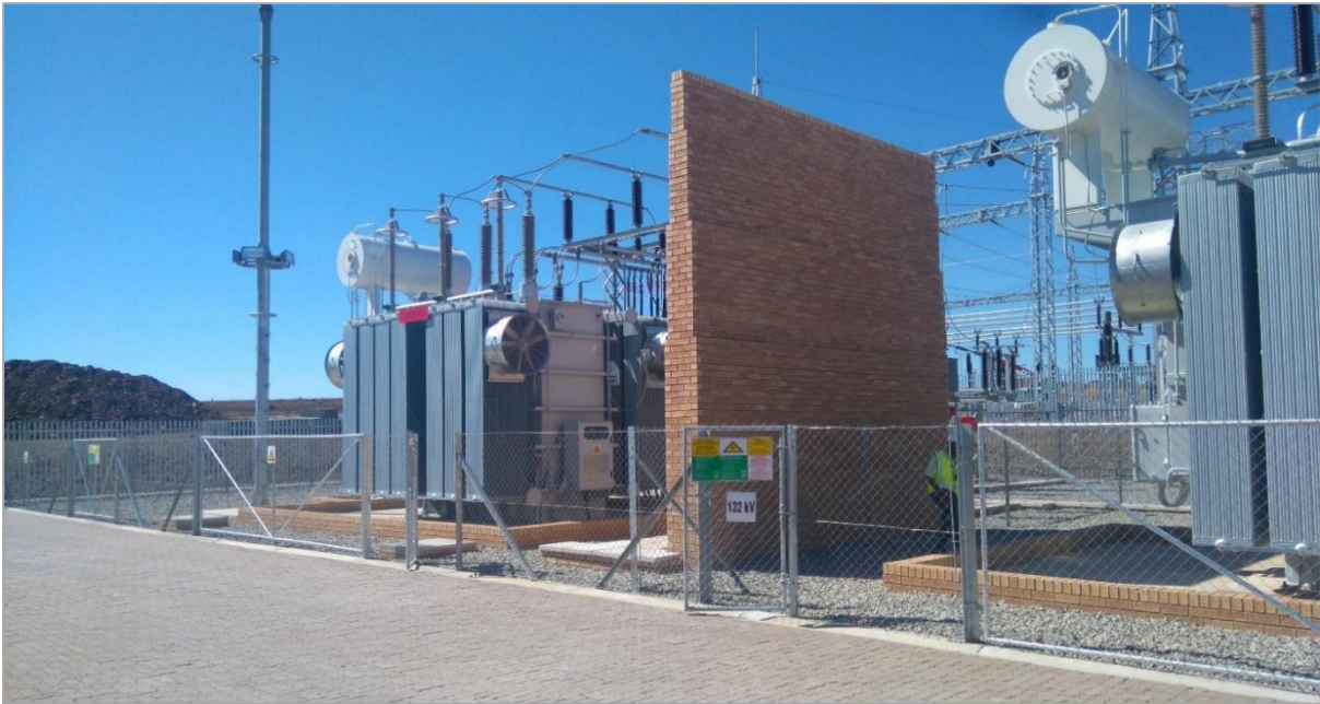
Figure 13: Example of High Voltage Transformers
