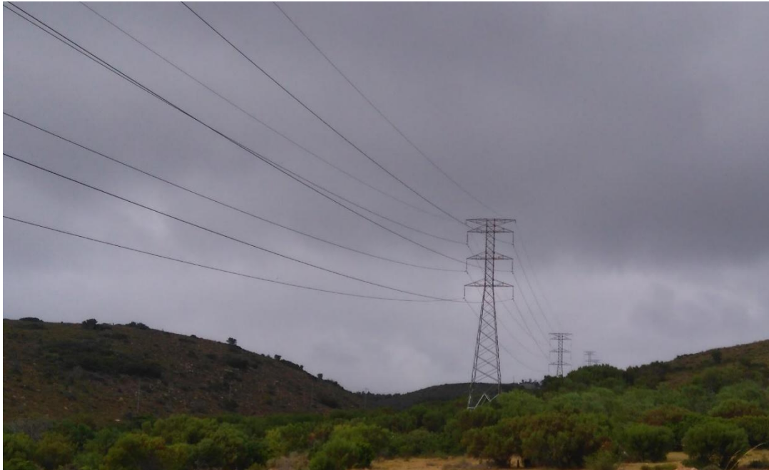
Figure 16: Example of a 132kV transmission line
