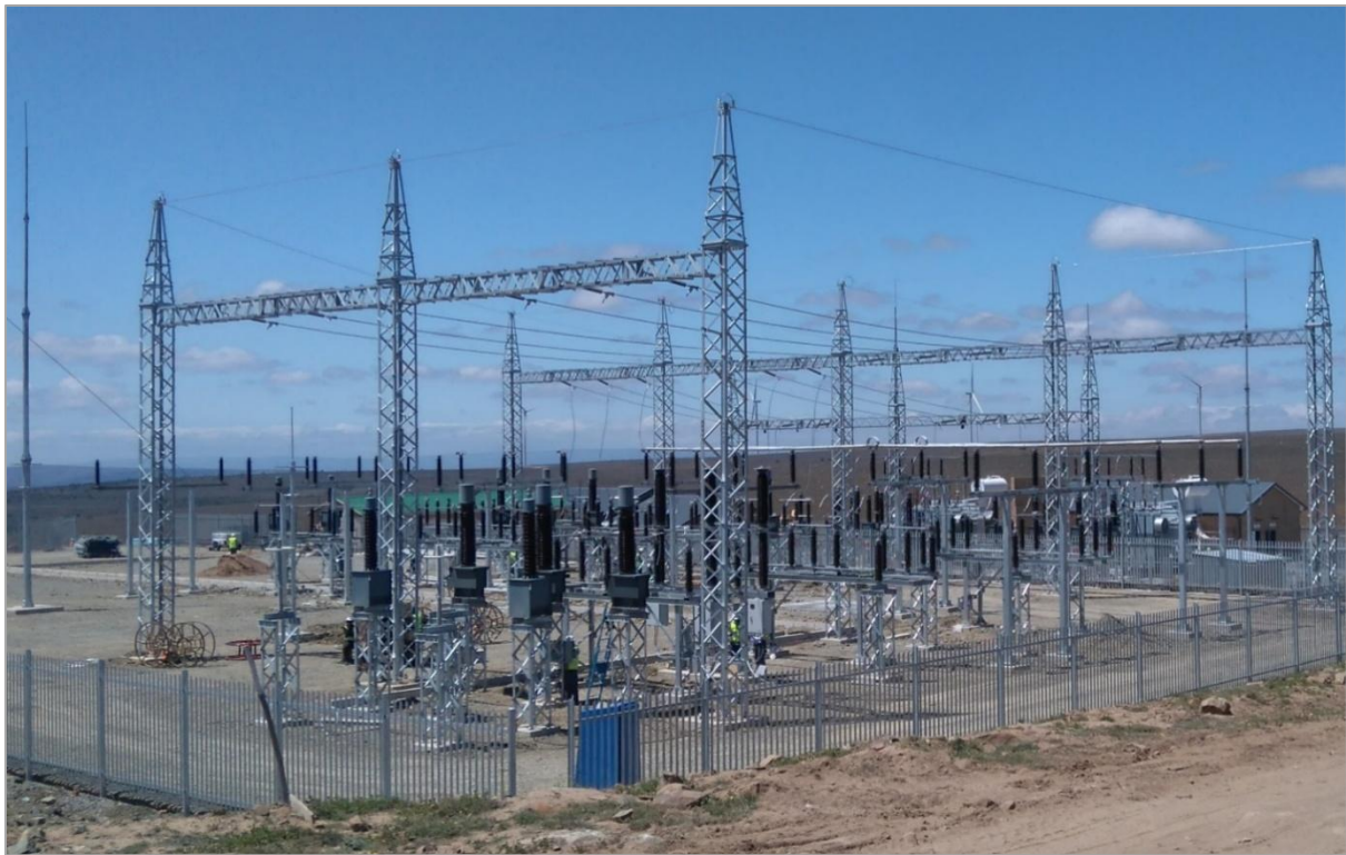
Figure 12: Example of High Voltage Substation
